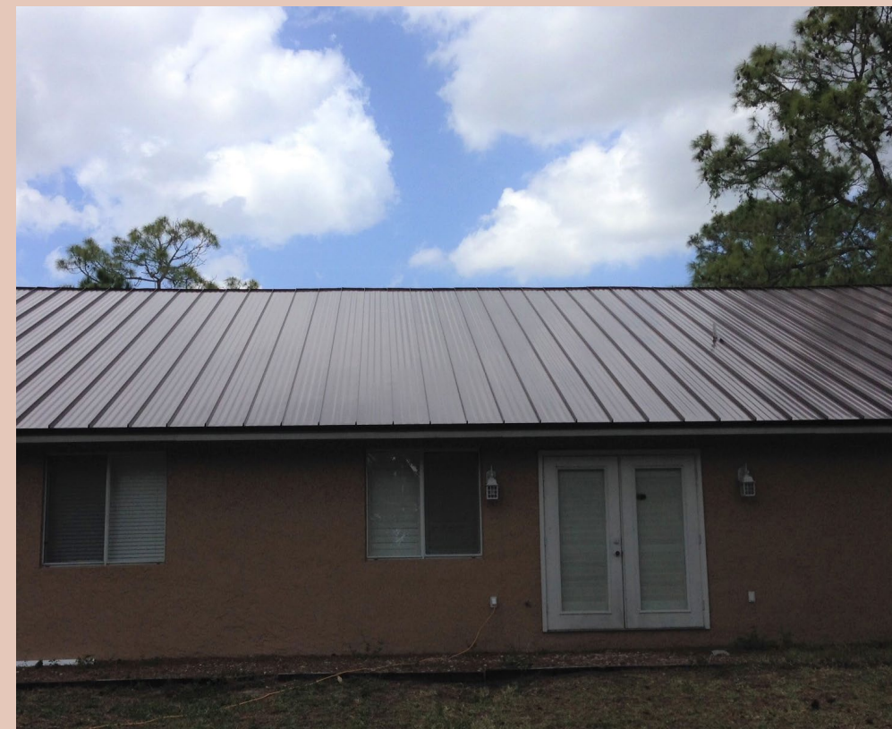
Timely Upgrade. Shortly after this inferior quality roof in Naples, Florida was replaced, it withstood Hurricane Irma with no damage.
