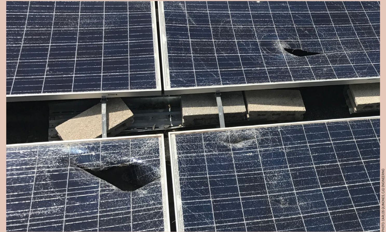
Rough ride. PV panels are often damaged by flying pieces from other panels.
